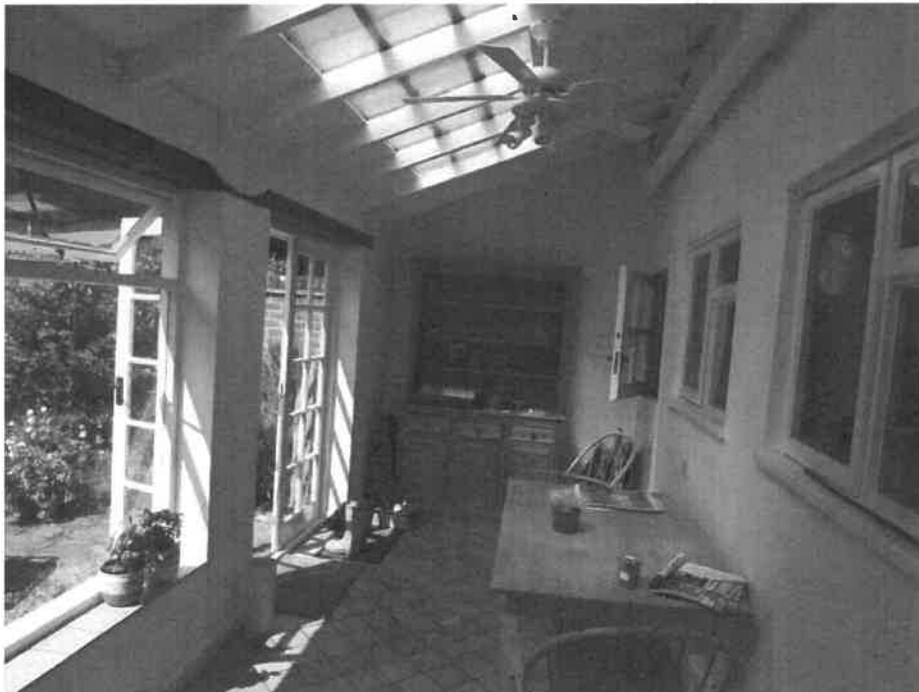
Inside original extension. Note no insulation and plastic roof sheets
